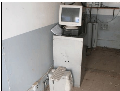
Inside the repeater building. That's the repeater under the monitor.
