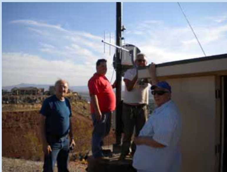
W7WFW, KE7MMH, K6LGA And KE7DZI at Work on Link Antenna to Toquerville Hill
